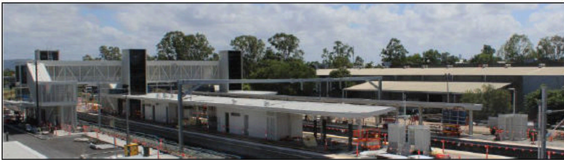
Work at Rocklea station is progressing with fit out of the station overpass and lifts, station buildings and canopies continuing.
